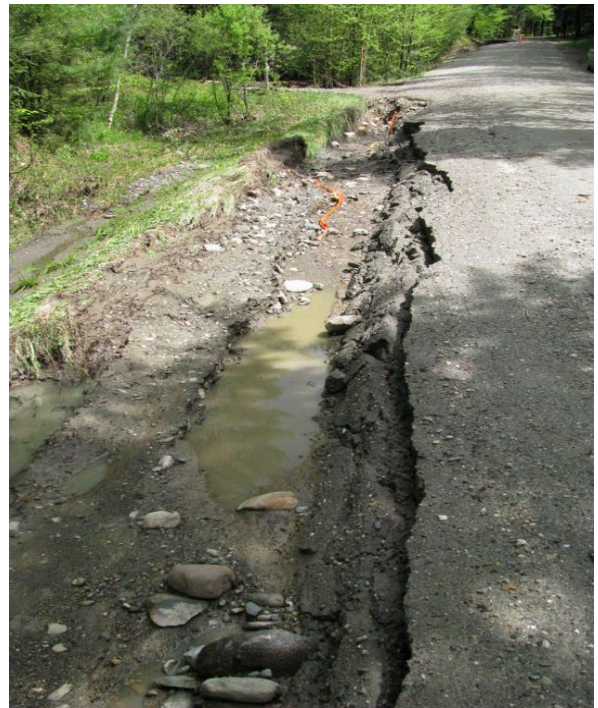
Brook Road Storm Damage – May 2011
