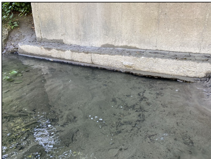
Abutment #1 Footing Undermining
