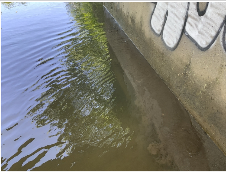
Undermining under abutment 1
