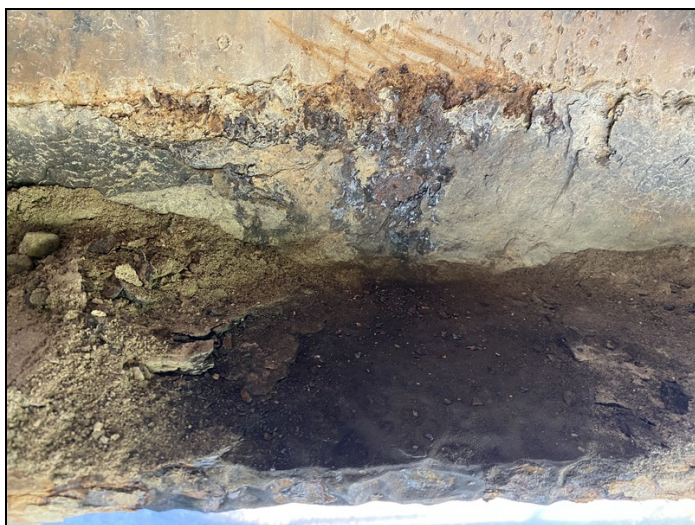
Pitting on Girder #2 Web at Floorbeam #3
