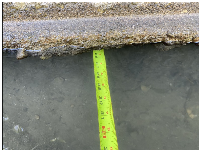
Abutment #1 Footing Undermining Penetration
