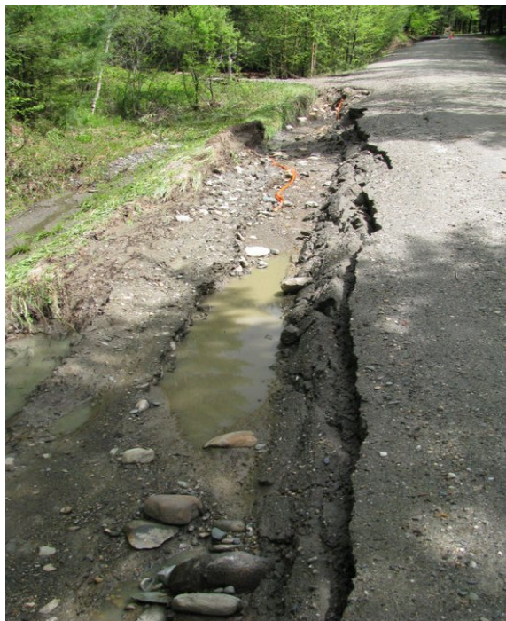
Brook Road Storm Damage – May 2011
